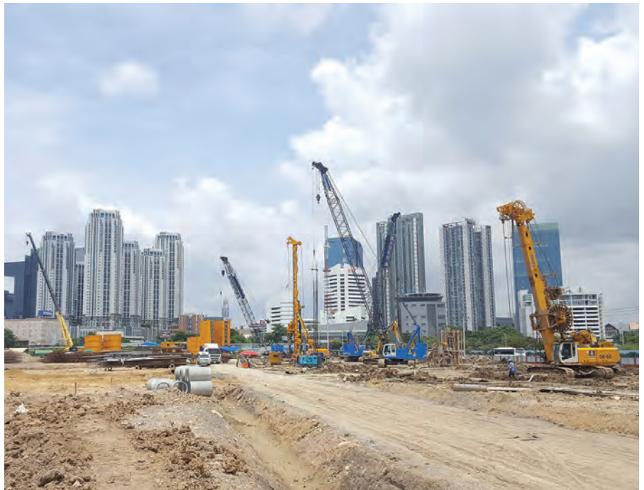
Thai Bauer carries out specialist foundation engineering works for the new MRT Orange Line in Bangkok. More than 370 bored piles with diameters of 800 to 2,000 mm are being drilled to a depth of between 40 and 65 m, and about 58,600 sq m of diaphragm wall with a width of 800 to 1,000 mm are being constructed down to a depth of 27 m.
