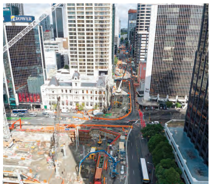
TOP AND ABOVE: A view of the Auckland City Rail Link (CRL) project. When completed, it will become New Zealand's first underground passenger railway and expected to ease traffic congestion.
