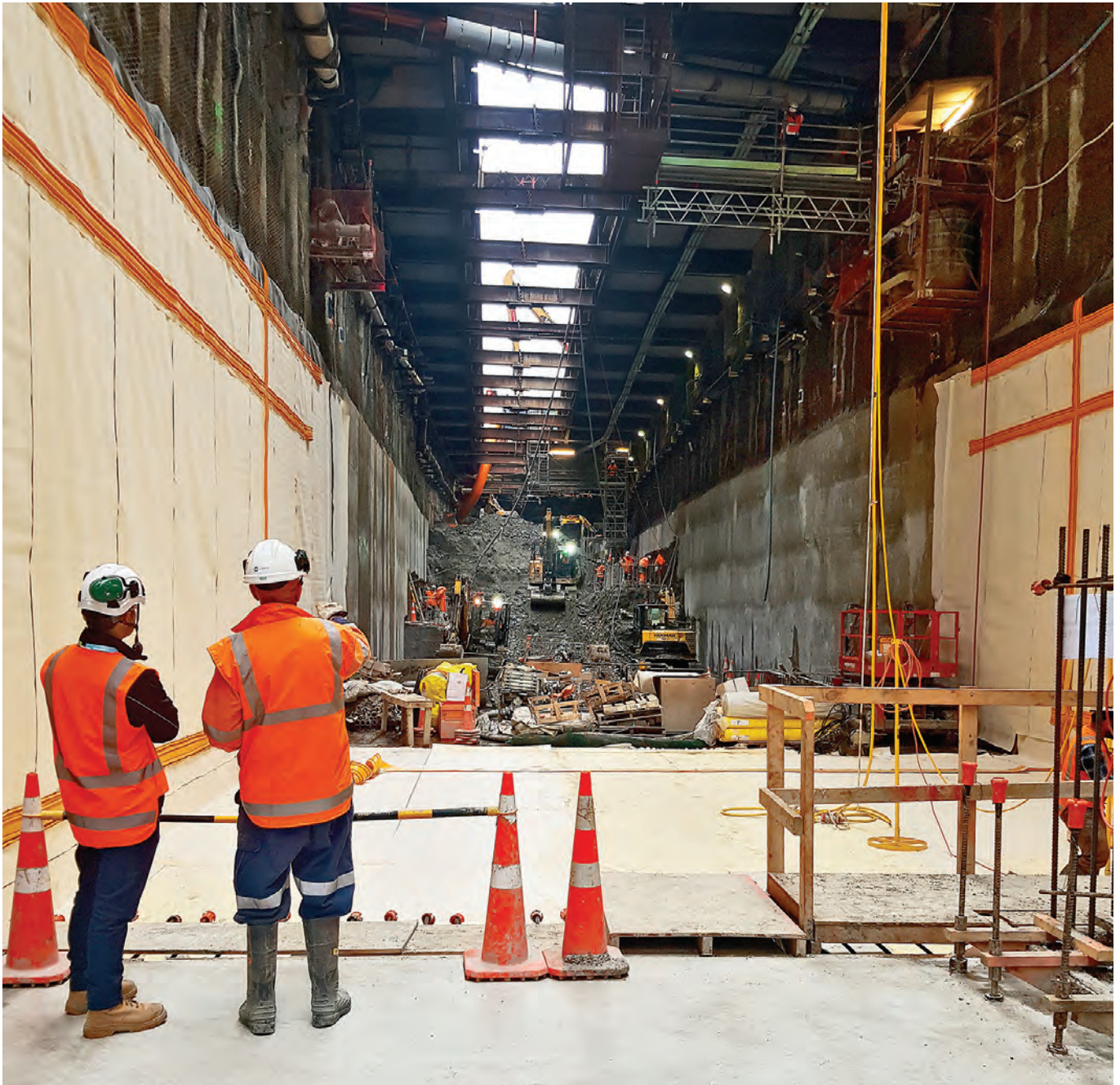
Construction of the CRL is still ongoing, and the project is scheduled for completion in 2024.
