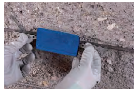
TOP AND BELOW: Mapeshield I being applied on a structure under repair.
