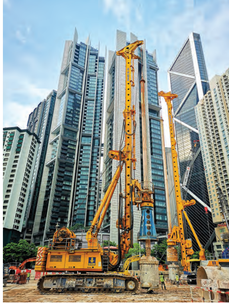
RIGHT: A Bauer BG 72 drill rig, equipped with a five-fold Kelly bar, is used to install piles up to a depth of 150 m.
