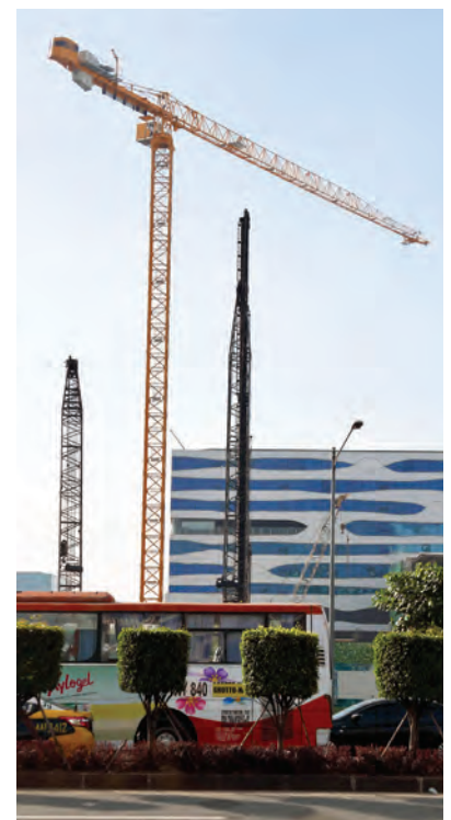
Whiteport has bought Potain MCT 205 tower cranes for use in a range of projects around Manila, the Philippines.
