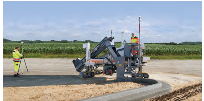
With the Wirtgen AutoPilot 2.0, the Field Rover measures the virtual string line support points.
